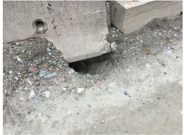
Fill erosion noted downstream left approach
