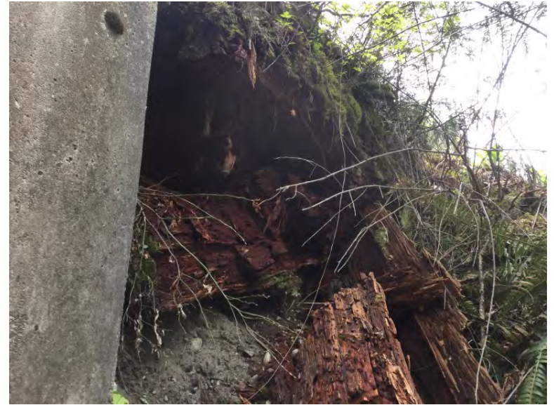
Rotten log retaining fill downstream left bank
