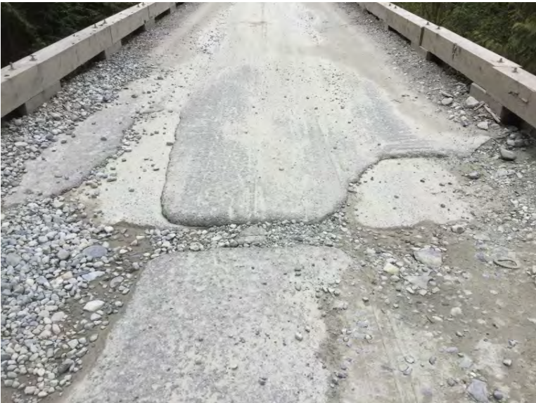
Asphalt overlay is wearing at right approach
